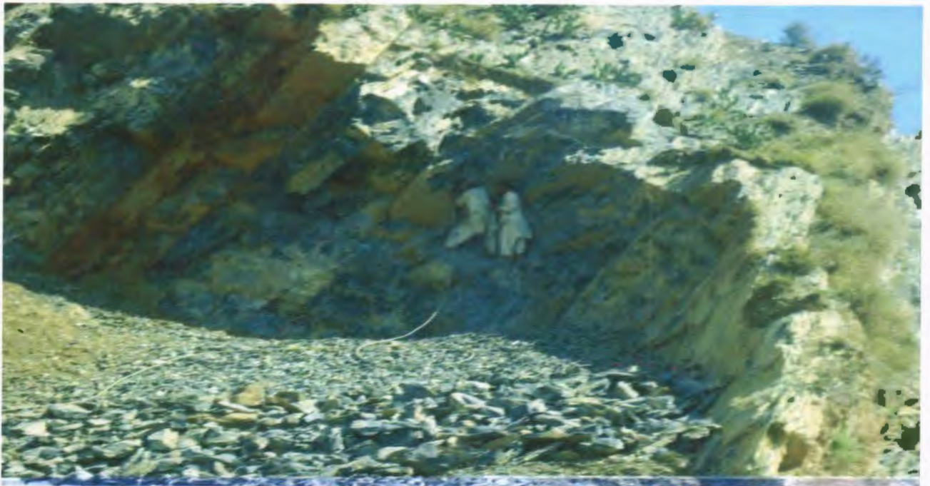
The two poor persons cut the hill with cutter to collect the stone for construction which earn money which is a threat to environment in Kala village.
